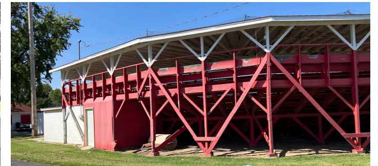
The full wooden structure can be seen from the back of the stadium.
